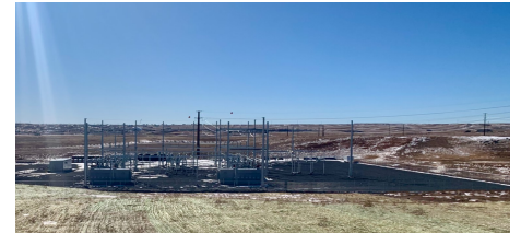
Orchard Valley 115kV / 13.8kV substation completed as part of Black Hills Energy's Ready Wyoming electric transmission expansion project
