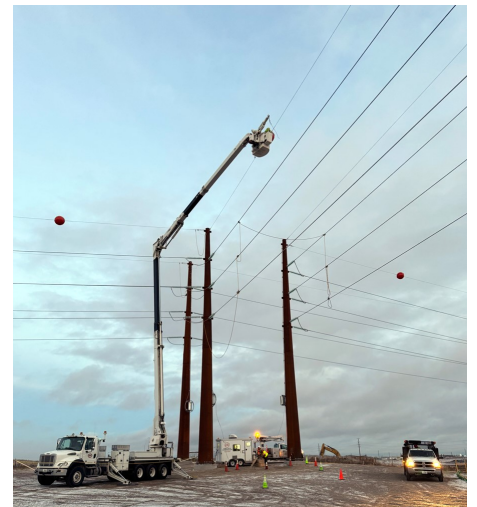
Construction on 115kV lines near Cheyenne, Wyoming as part of Black Hills Energy's Ready Wyoming electric transmission project
