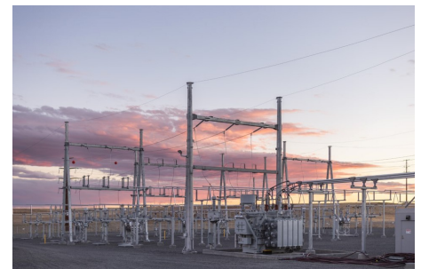
Ready Wyoming - Orchard Valley Substation
