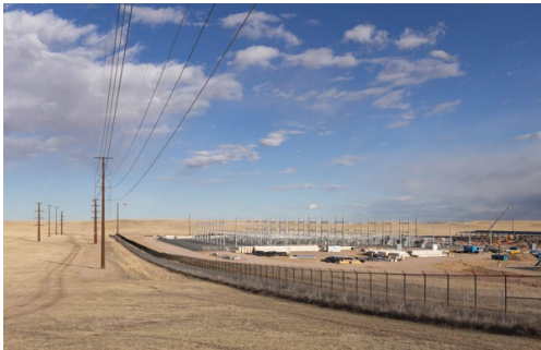
Pictured: Bison Substation and Ready Wyoming transmission lines
