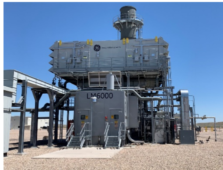
Figure 05-2. Cheyenne Prairie Generating Station Simple Cycle CT
