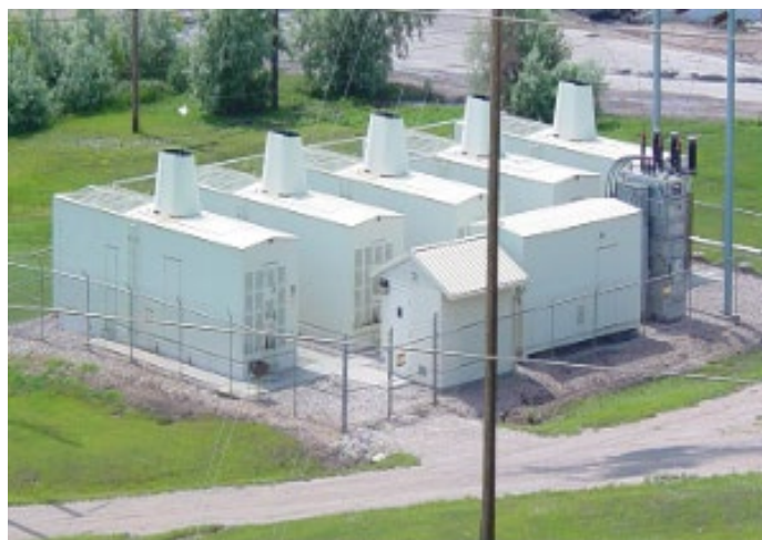
Figure 05-3. Ben French Diesel Generators
